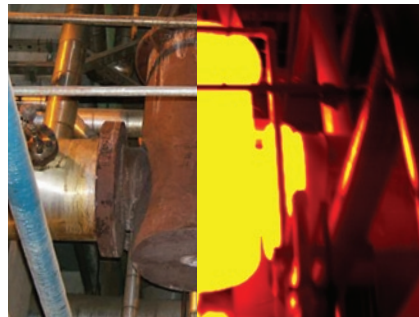
28" Diameter high pressure steam pot (operating temp 650°F) located in the kraft mill. Real photo on left, thermal image on right. Bright yellow indicates the temperature of the vessel and can help determine any radiant heat loss.
